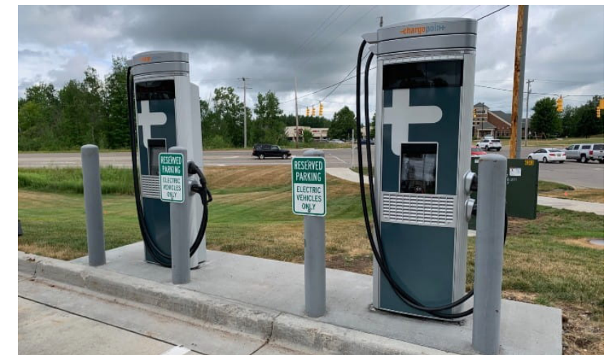
An example of EV charging stations
