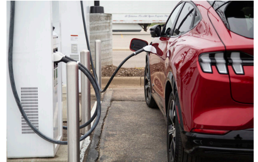
An EV Charging Station
